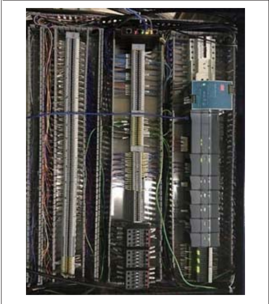
FIG.3. PLC control panel
