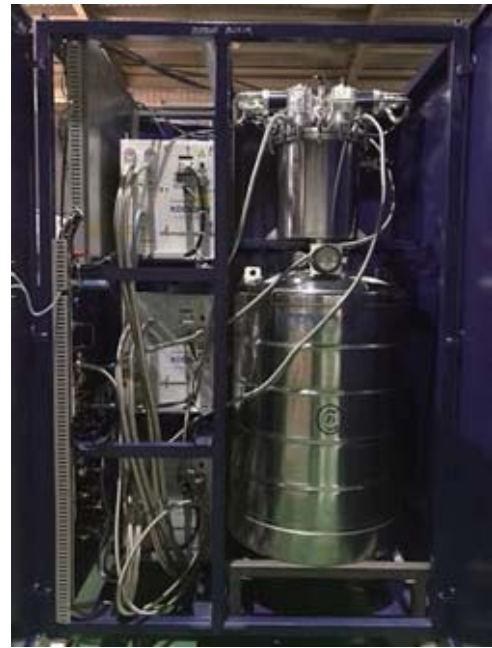
FIG.7. The whole liquefier system
