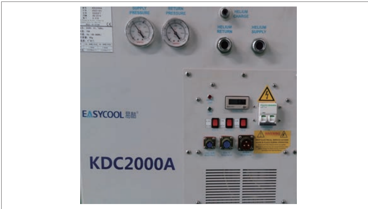
Figure 5 Electrical Control Panel
